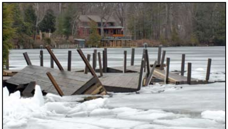
Overuse of ice eaters to protect docks can actually cause dock damage!
