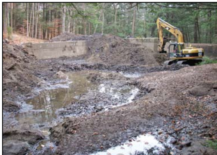
Almost 600 cubic yards of material were removed when Hubble Brook Reservoir was cleaned out this past October.
