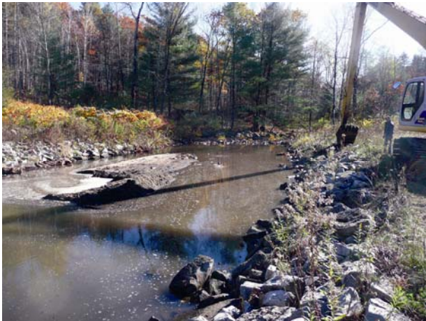
Photo caption: Last week, crews cleaned out the sediment that has built up in a retention basin on Hague Brook. This pond on the upper part of the brook was originally constructed by the LGA in 2006. Over 45 dump-trucks full of material was removed from two different retention basins on the brook.
